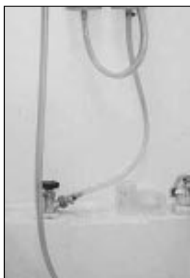
Figure 2 - De-ionised water system at R&R
